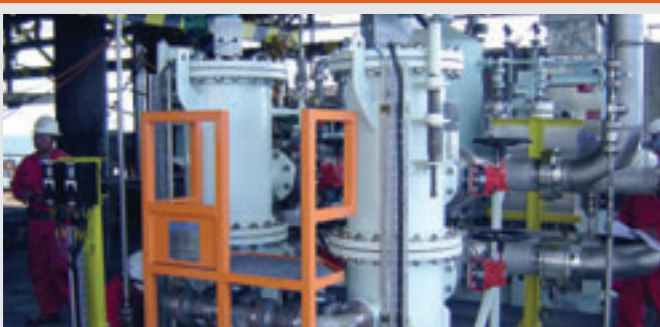
Water injection Malaysia offshore, 280 m 3 /hr, 40 micron
