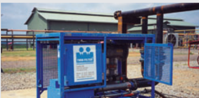
Produced water re-injection Sumatra, 30 m 3 /hr, 25 micron
