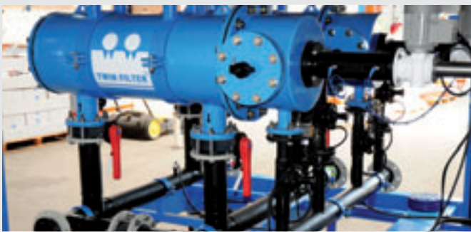
Seawater Intake 700m 3 /hr at 50 micron, housing carbon steel rubber lined, SM0254 internals Piping HDPE, Controls Eex-d
